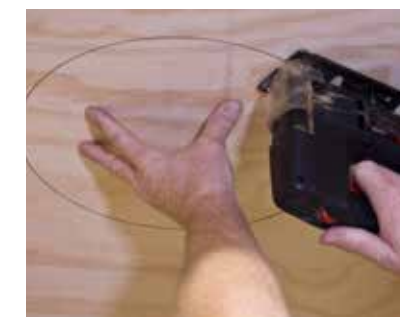
8. Drop a plumb line from roof to center of chimney. This establishes the center point for cutting a round hole through the roof.
