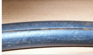
Failed pipe seam covered under warranty
