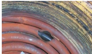
Pipe rupture due to freezing or obstruction
